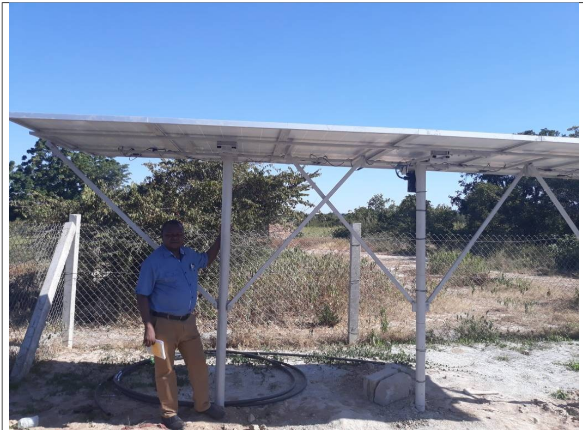
Fig. 4: A solar panel in one of the three water projects implemented by TADELO in Kurio village, Chemba DC
